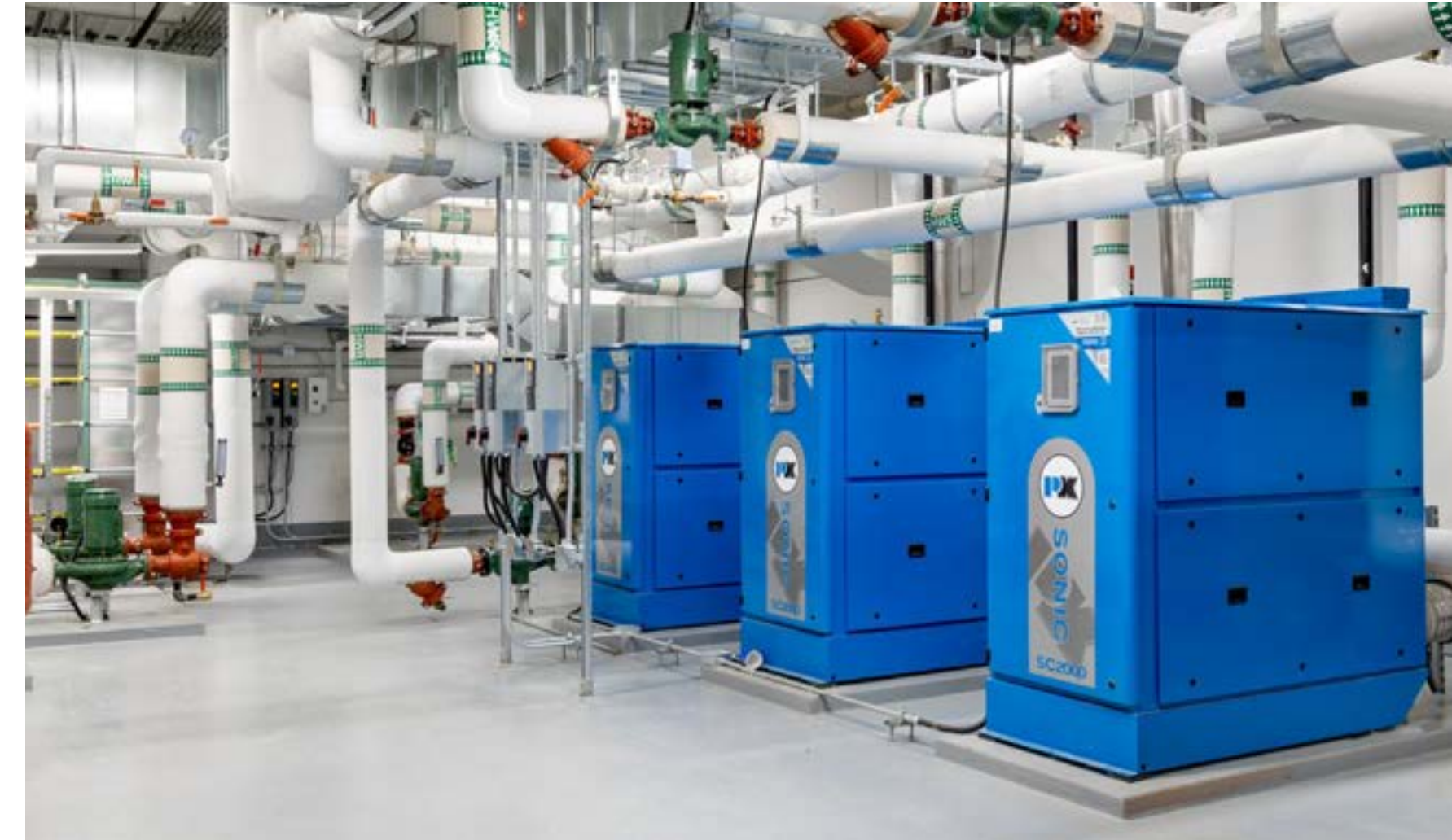
Mechanical room at the Canadian Blood Services facility in Calgary
